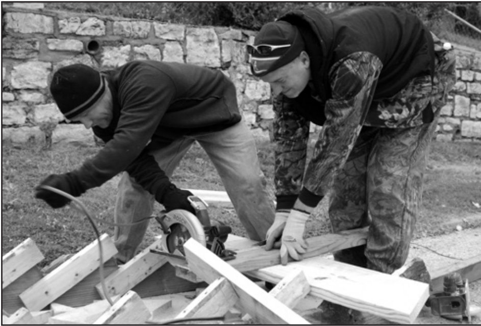
Christmas in October volunteers, pictured above working on the house of Tracy Aguilar, were happy to bear the cold air and provide assistance to some of the residents of Rosedale.
